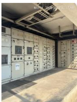
Electrical panel with rubber mat.JPG
