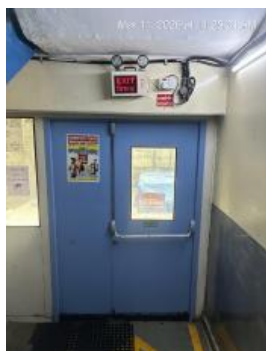
Emergency exit door.JPG
