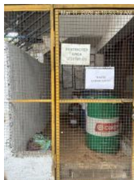
Oil storage room.JPG
