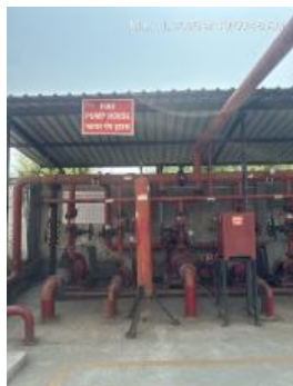
Fire Pump room.JPG
