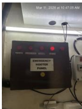
Fire Alarm call panel.JPG
